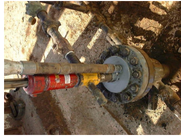
Annular well head with pressure control pack-off installed.
